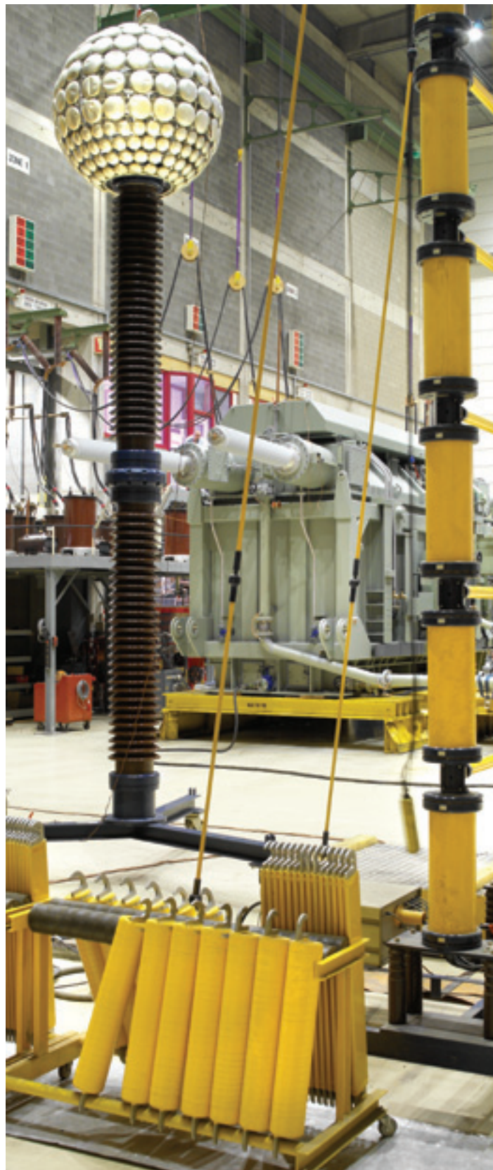
Testing environment for a 150 MVA 235/34.5 kV ODAF generator transformer with special tank construction according to German Rail standards >
