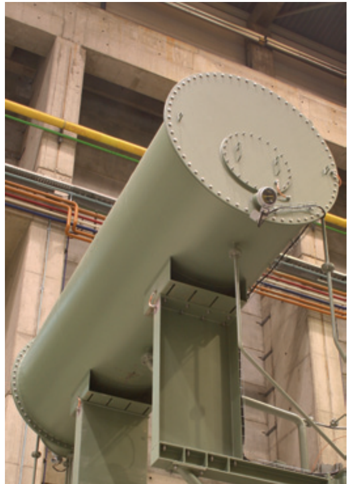
^ The conservator with oil level indicator for main tank oil at 30° angle
